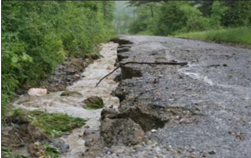
Stormwater degrades Monkton Road Photo credit: Buzz Kuhns.
